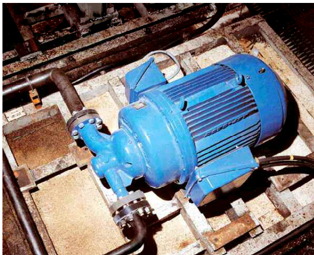
Figure 16. Variable Speed Pitot Tube Pump in Place at a Yorkshire, United Kingdom, Power Station.
