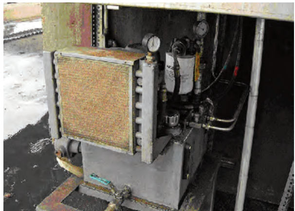
Figure 1. Circulation Oil System.
