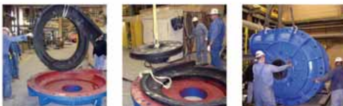
Three photos below: Sequence showing the fit up of a 400 MCR wet end
