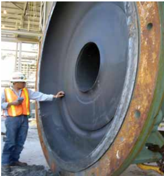
Pump casing liner and throat bush at 13 week inspection.
