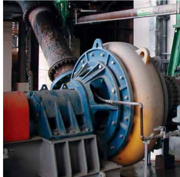
Warman 550 MCU unlined mill circuit pump in service
