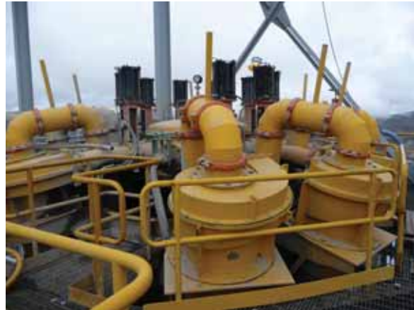
Typical hydrocyclone cluster
