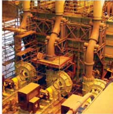
Right: Three Warman 550 MCR mill circuit pumps being installed at a copper mill along with Cavex hydrocyclones, Isogate slurry valves, and Vulco wear resistant rubber lined tanks, piping, hoses and spools
