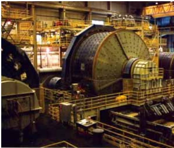
A typical SAG mill with a smaller conventional ball mill shown in the background
