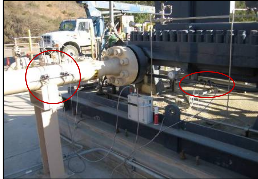
Dual traverse flow cells installed on the suction and balance line leak-off piping
