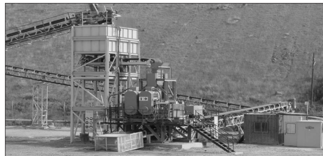
Figure 6. The pilot facility at Mogalakwena South
